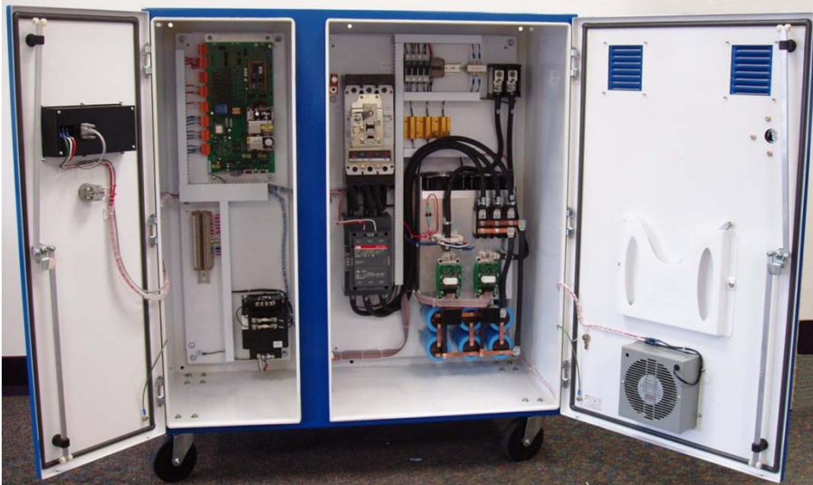
Mid Frequency 400 Hz Power Supply Control Cabinet
