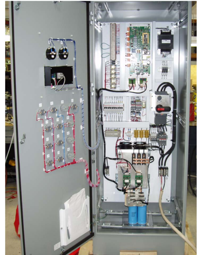
Mid Frequency 400Hz Power Supply Control Cabinet
